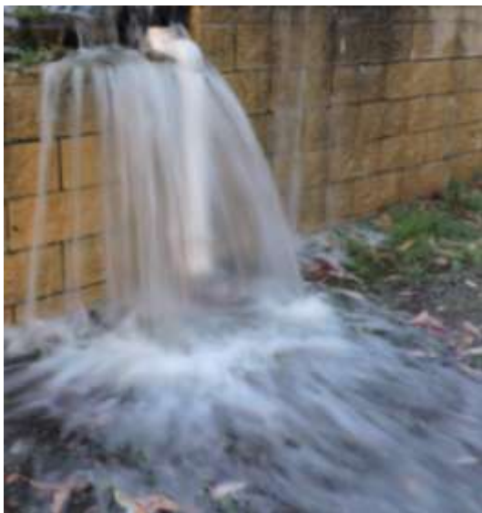
5-30 am New Year's Day Water line burst - water outside But non inside
